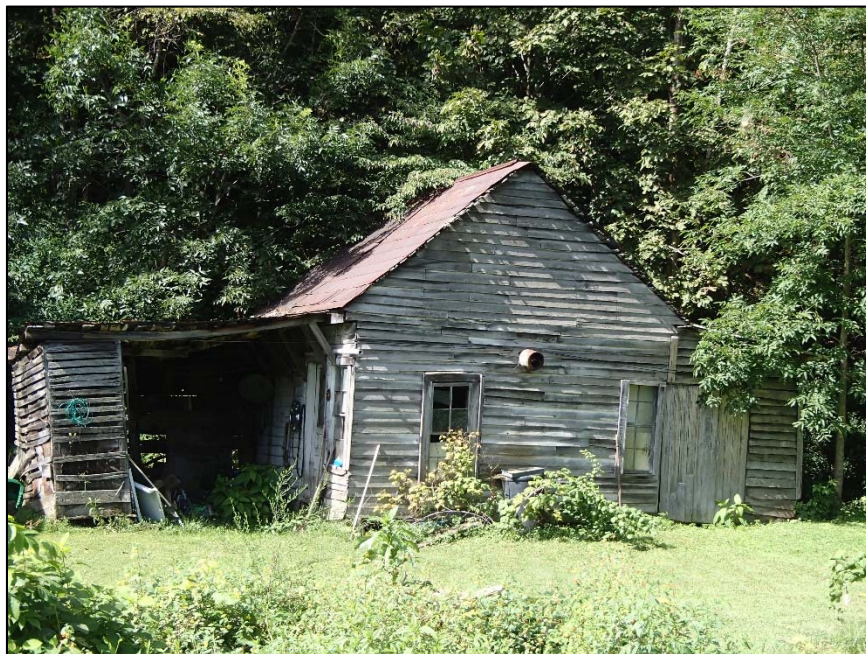
Figure 57: Eli and Minnie Oliver House, earlier house or kitchen as outbuilding, north elevation
